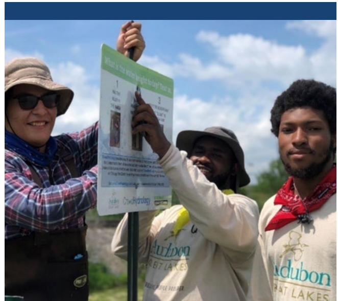
Installation of educational signage at Big Marsh Park, IL, by Audubon Great Lakes interns. Photo Credit: Teri Valenzuela/Audubon Great Lakes
