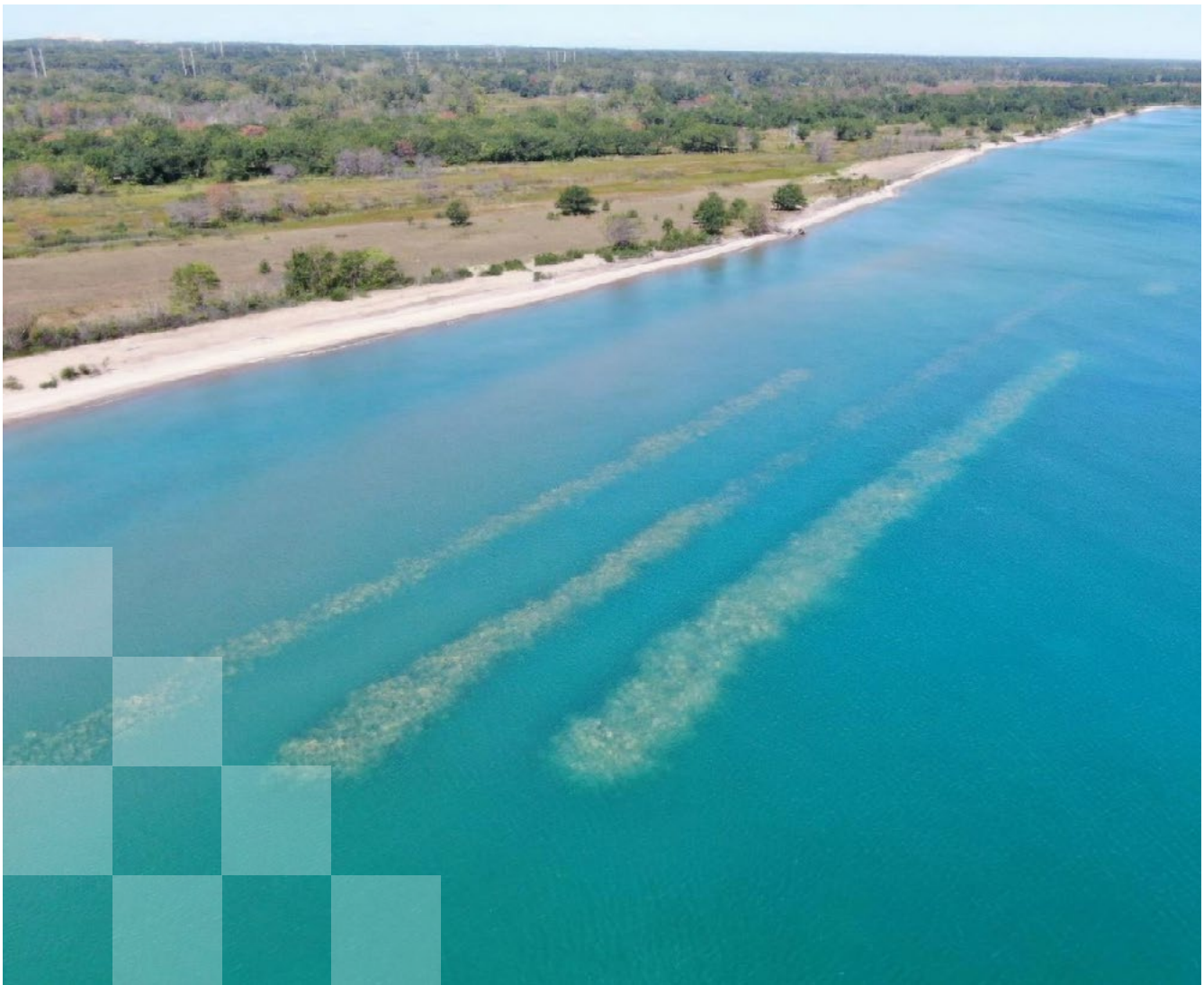
Aerial view of fully installed submerged rubble ridges at Illinois Beach State Park. Photo credit: US Army Corps of Engineers
