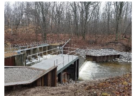
Completed sea lamprey trap at East Branch Au Gres River. (Credit: USACE)
