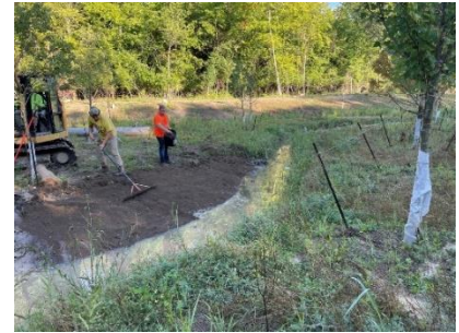
Active restoration work to correct stream channel alignment on Tamarack Creek. (Credit: Alliance of Rouge Communities)
