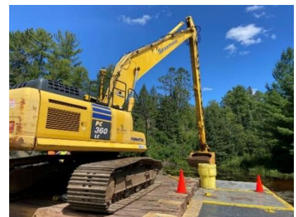
Placement of a sediment cap containing pelletized activated carbon mixed with sand to absorb and immobilize contaminants in Scanlon Reservoir. (Credit: USACE)
